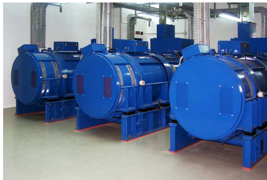
Mechanical UPS – uninterrupted drive of rotating Machines (e.g. pumps).
